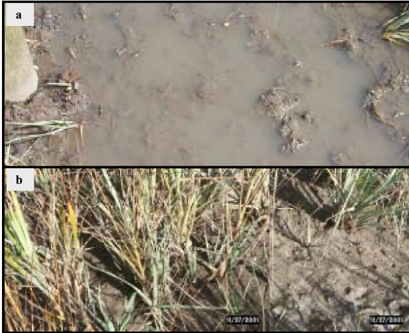
Figure 13. Photographs of the area adjacent to a dock during the construction phase (a) and approximately one year after the construction (b). The photograph during construction was taken on August 7, 2000 and is to the right of the dock walkway. The photograph post-construction was taken on November 27, 2001 and is to the left of the dock walkway.
